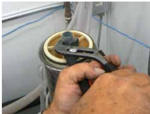
After the collar is off, grab the nipple on the filter with your plumber's pliers and turn and pull at the same time.
